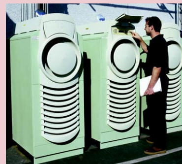
Multiple microturbine installation.
