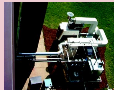
Cogeneration at the University of Maryland consists of a microturbine and a small capacity direct-fired absorption chiller/heater.
