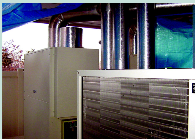
Figure 4: Microturbine and exhaust-driven air conditioner.
