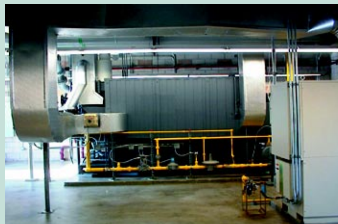
Figure 6: Inside the chiller/microturbine plant. View shows the absorber (center) and microturbine (right).
